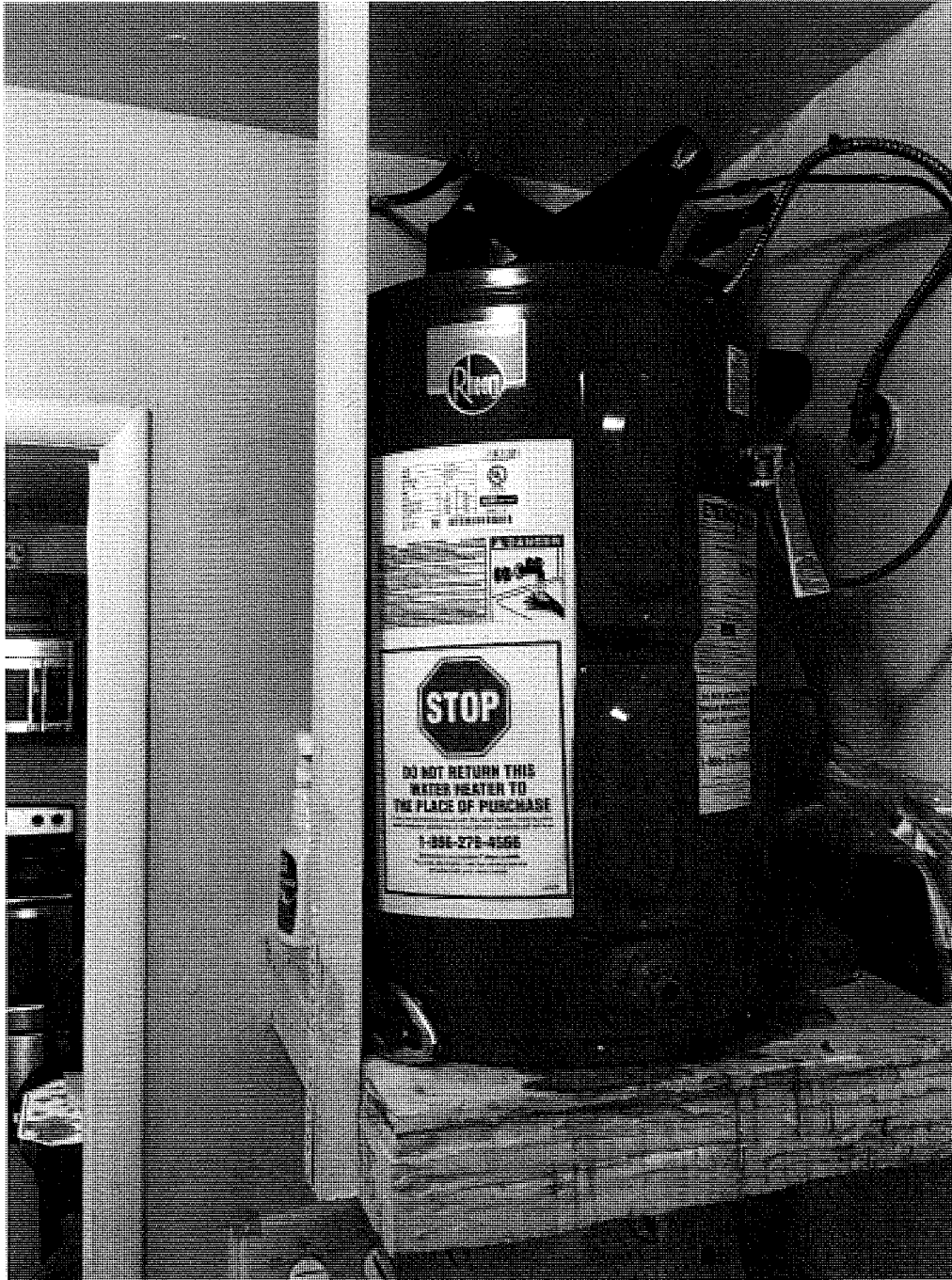
Domestic Water Heater
