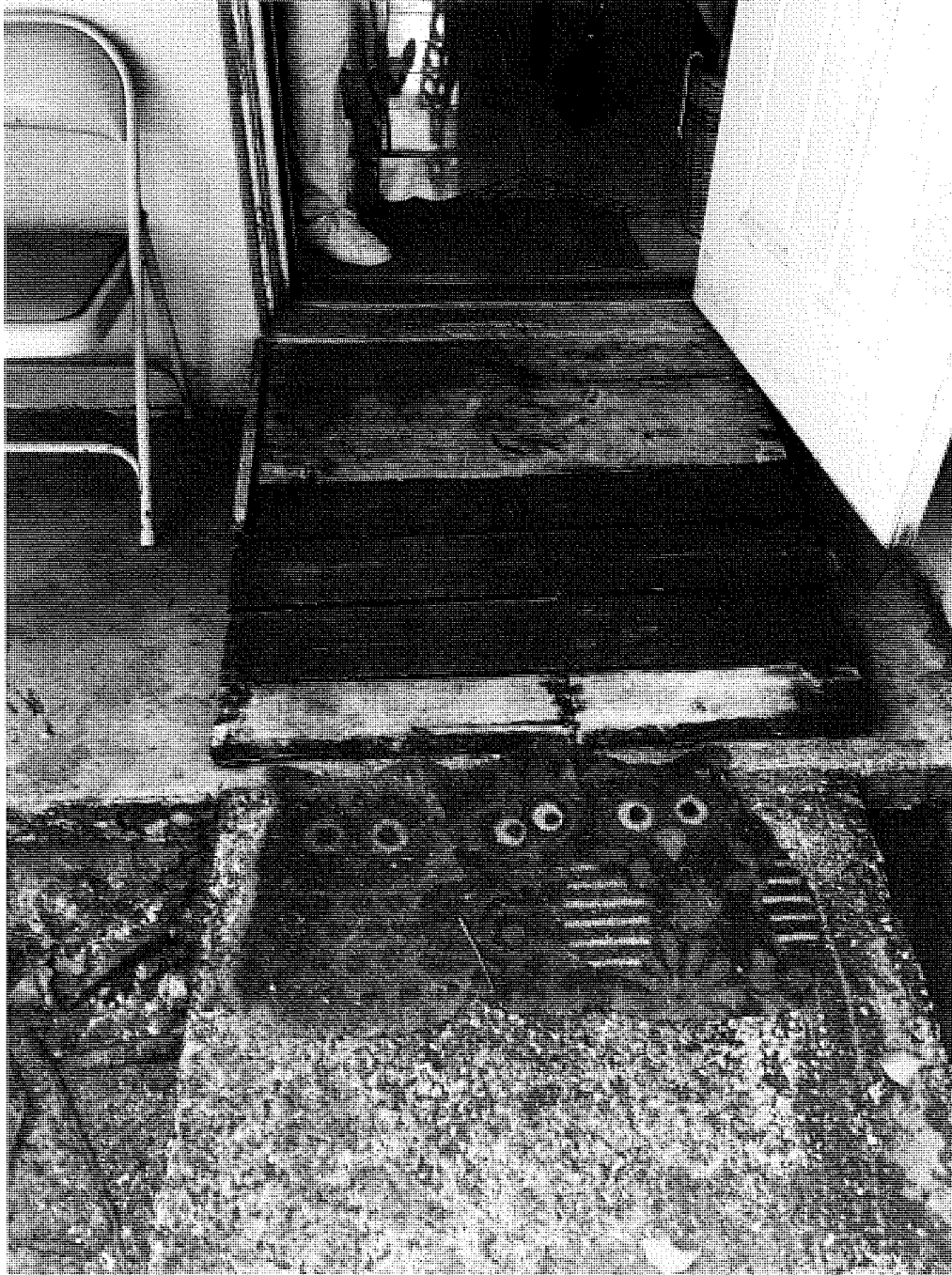
Entry Ramp in disrepair
