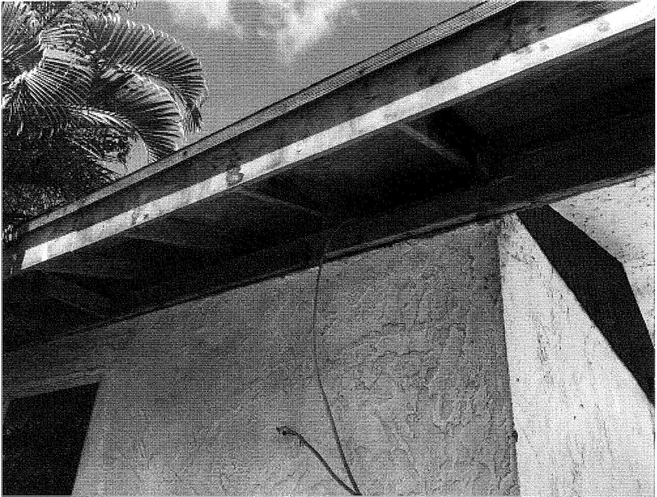
Exposed Electrical wiring at exterior
