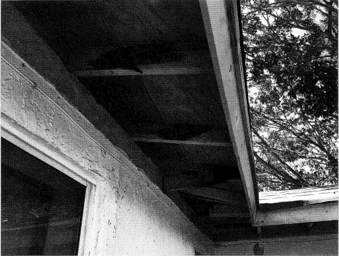
Ceiling exposed to the atmosphere due to lack of proper soffit and fascia boards. Also note the signs of rotting on the trusses.
