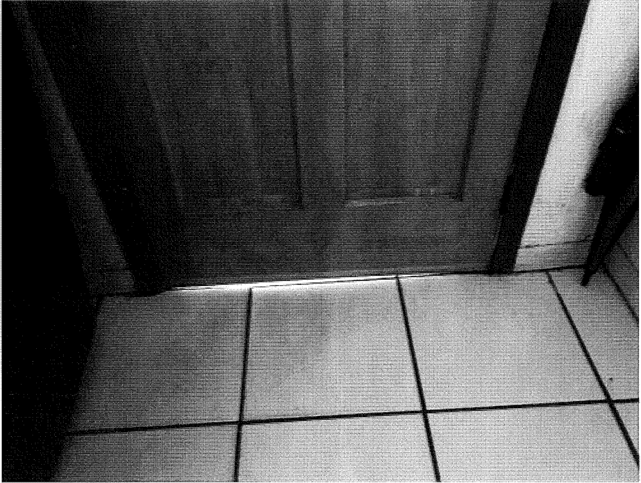
Undercut at Front Door
