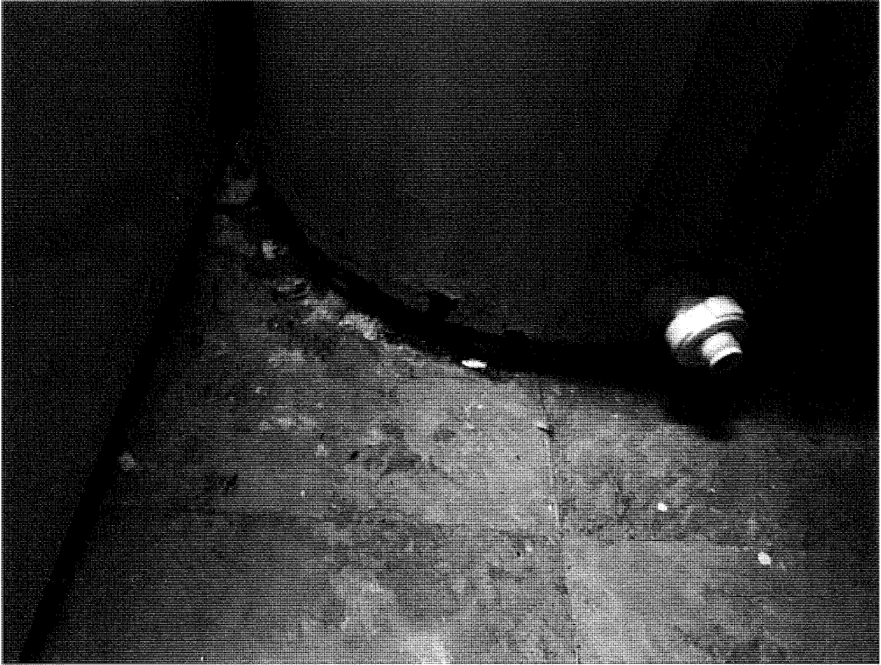
Domestic Water Heater
