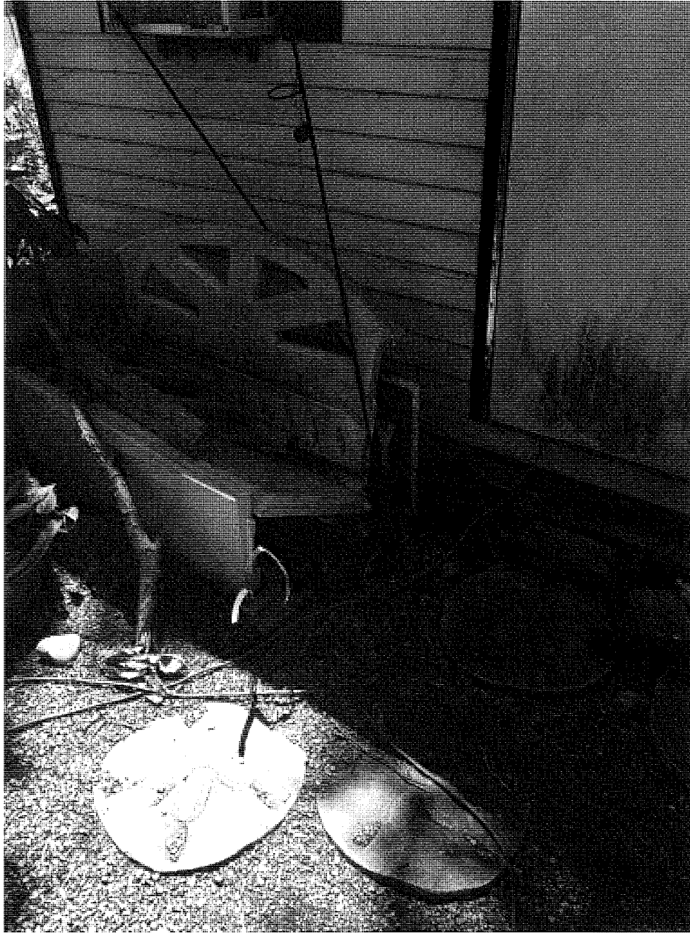
Extension cords being used to supply power to shed in the backyard
