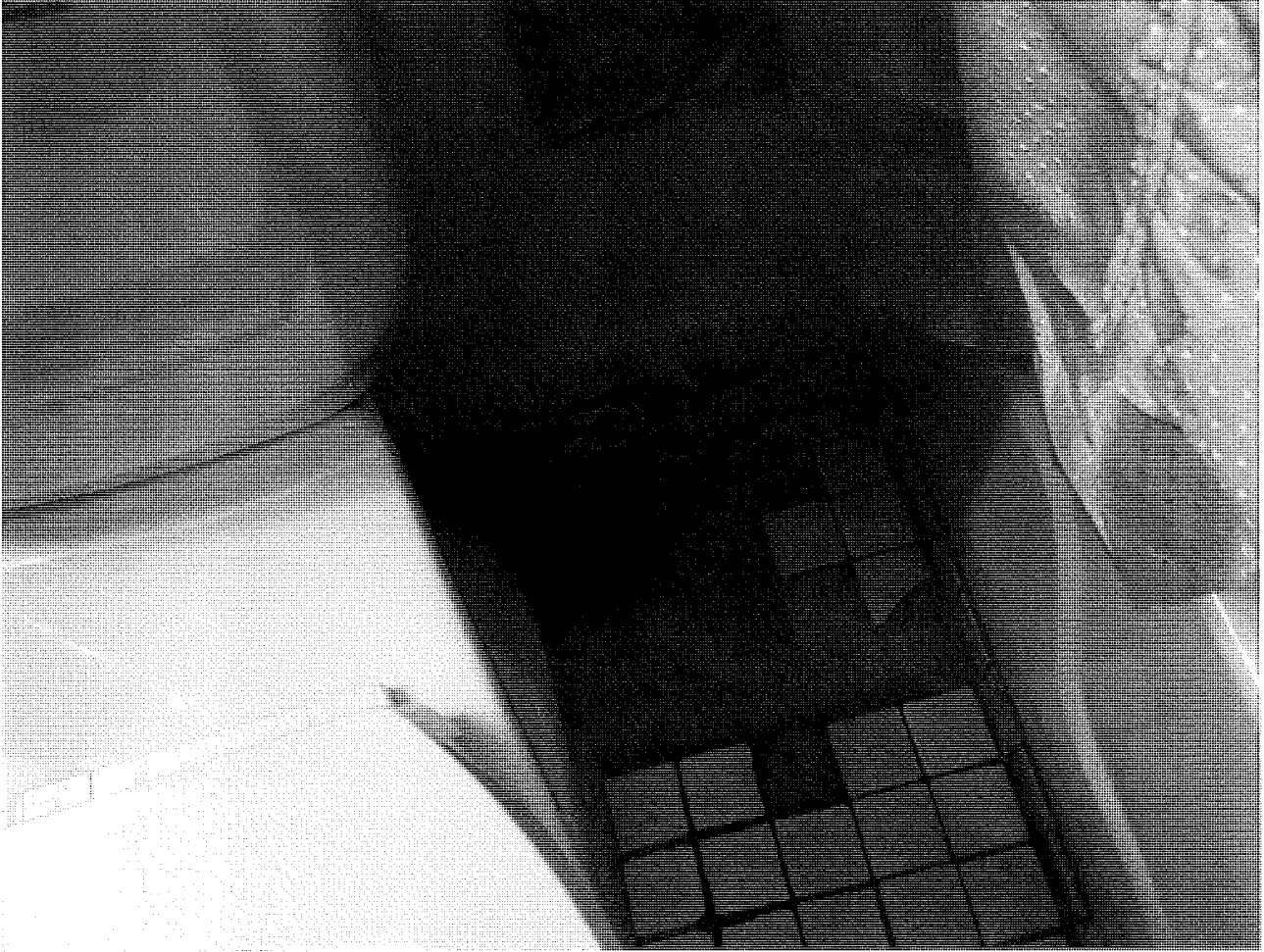
Damaged Wall at Master Bathroom
