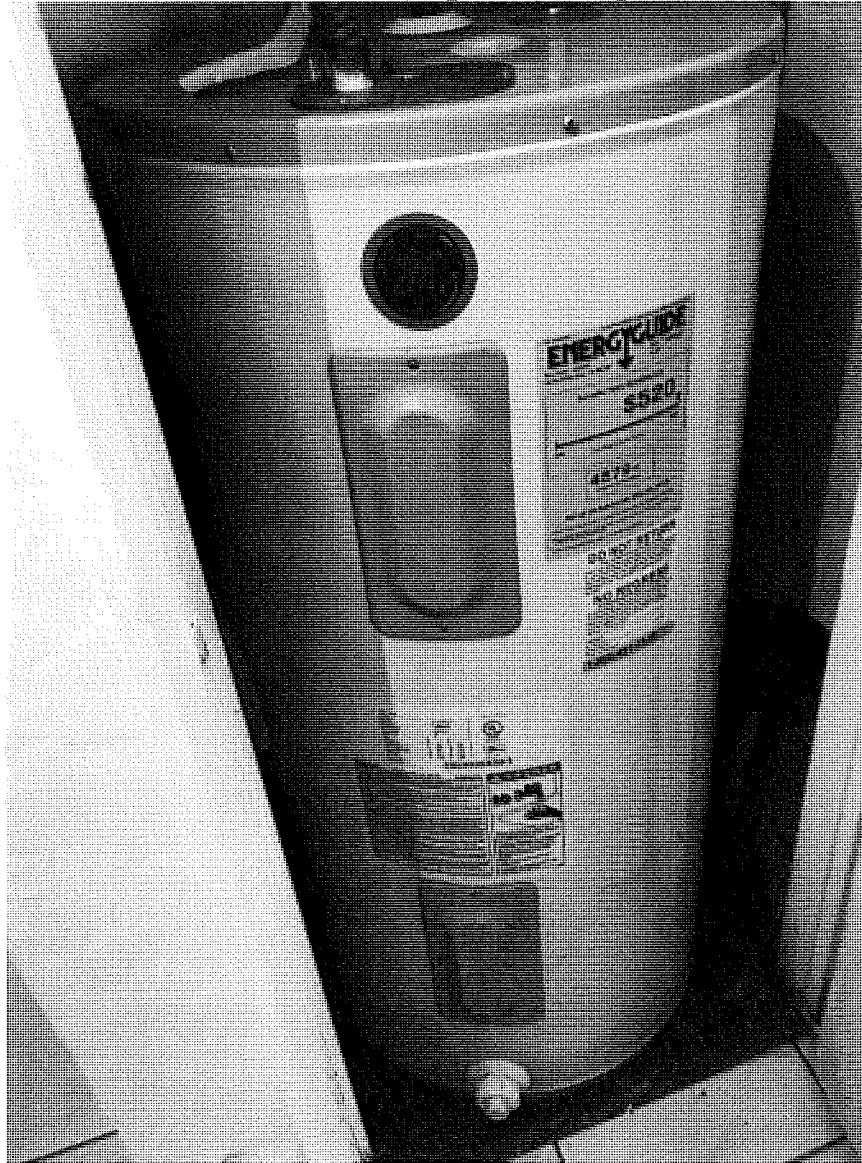
Domestic Water Heater
