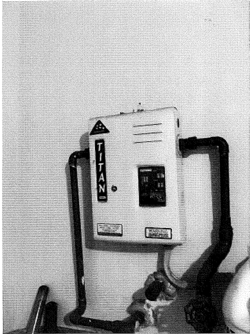
Domestic Water Heater
