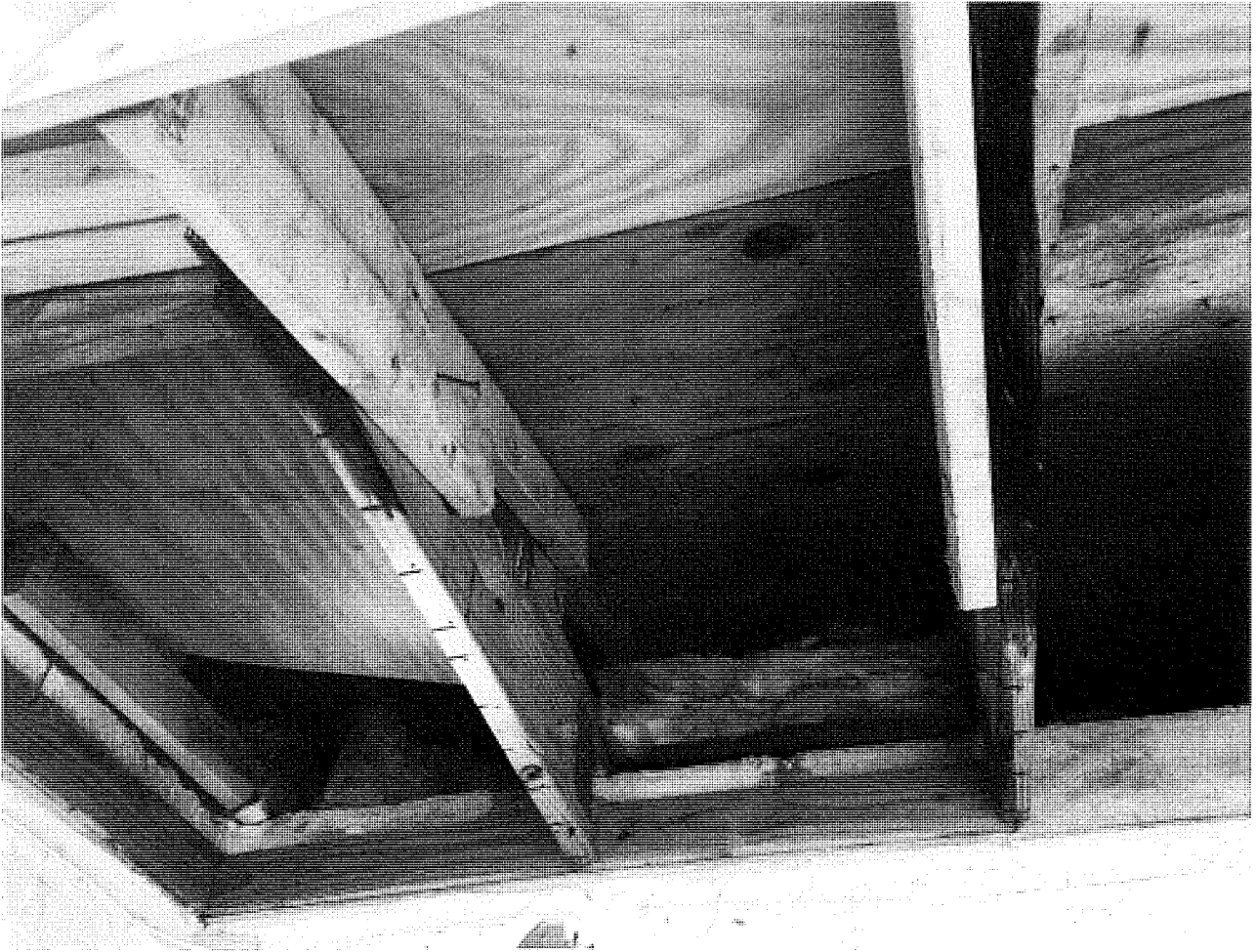
Ceiling exposed to the atmosphere due to lack of proper soffit and fascia boards. Also note the signs of rotting on the trusses.
